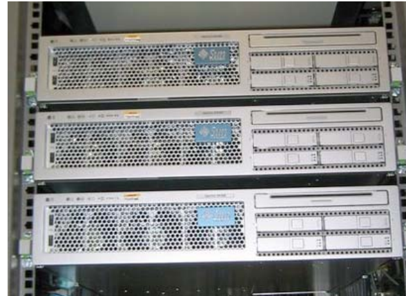
three X4200 for services (grid, batch, web, monitoring, gridftp)
