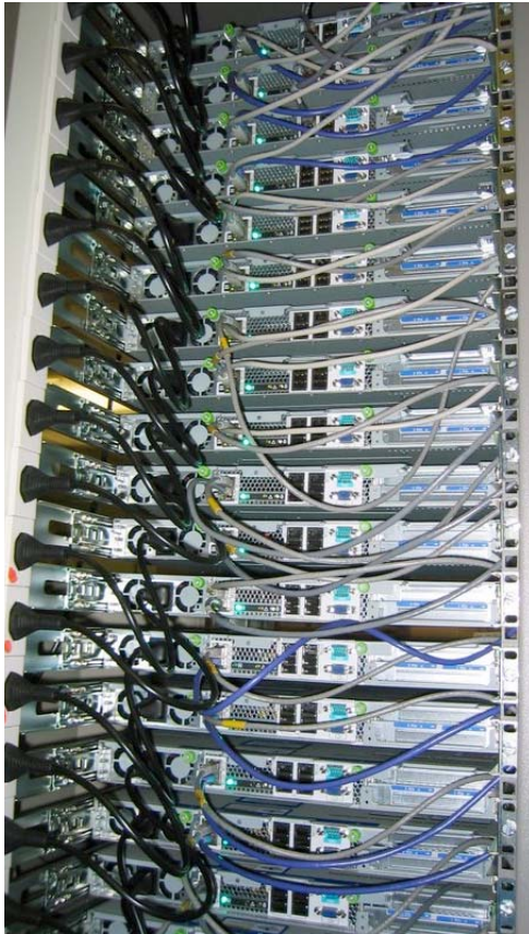
power and network cabling of worker nodes
